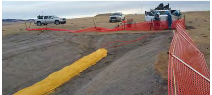
Deployment in the field
