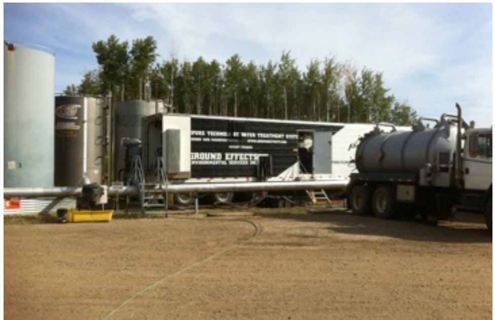
Ground Effects Environmental's mobile treatment set-up will virtually eliminate the need for trucking waste water off-site.
